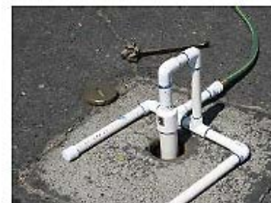
Discharge to cleanout
